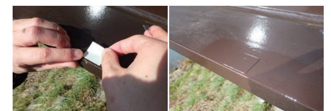
Simply remove the rust, apply the sheet, and paint the top coat.
