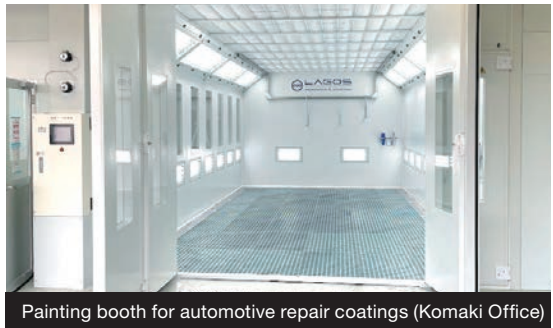
Painting booth for automotive repair coatings (Komaki Office)
